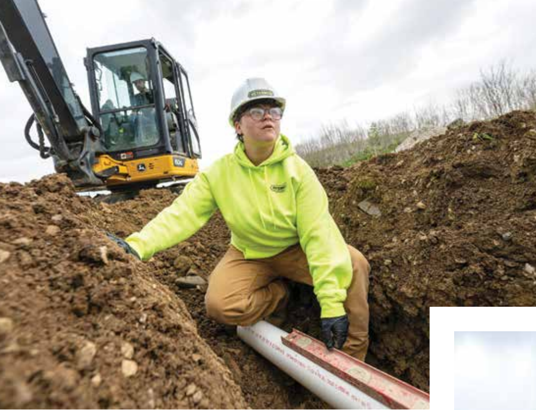
« Layne Pullium levels a section of pipe while Tyler Peterman operates the John Deere mini excavator.
