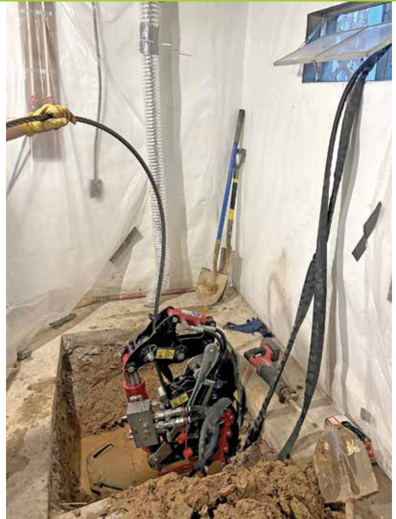
It took only 13 minutes to draw the 100-foot length of 4-inch replacement pipe into place using the lateral pipe bursting machine. Power was supplied using a dedicated hydraulic powerpack.
